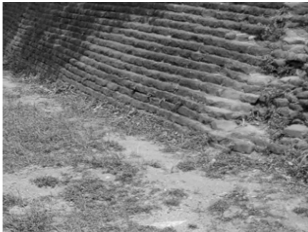
“Figure 03: Deterioration of brick walls due to visitor’s foot. (Pushpa Kumara, 2024)
